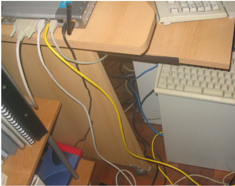
Figure 11 - HUB2 connections after handover.
